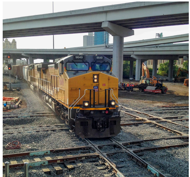
UP 9649 pulls the first train across the upgraded interlocker Aug. 28, nearly two weeks ahead of schedule.
