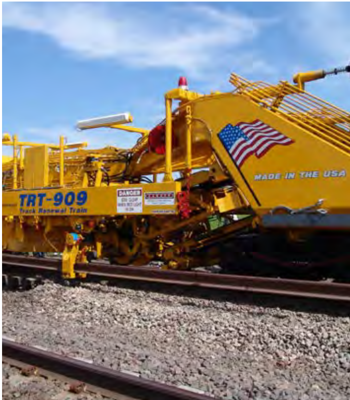
Union Pacific used equipment such as its track renewal train to replace more than 4 million railroad ties in 2012.
